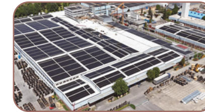
4.4 MW ELKA PV system
