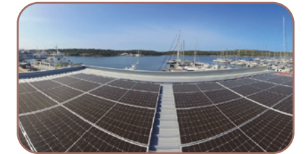
0.75 MW Iskra Shipyard PV system
